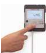
HMI control system on wall
